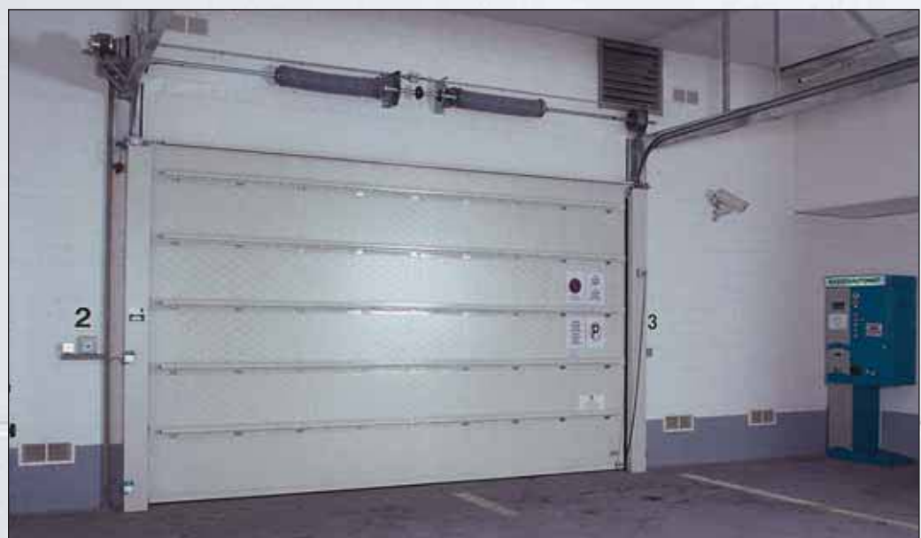
T30 Sectionaltor in Tiefgarage.
